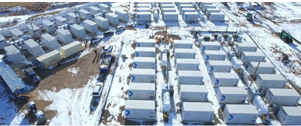
Hithium Colorado Energy Storage Project
