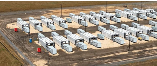
Hithium Texas Energy Storage Project
