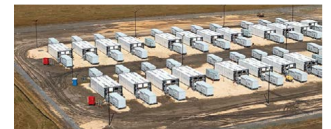
Hithium Texas Energy Storage Project
