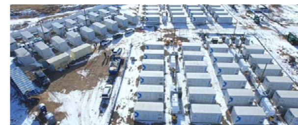
Hithium Colorado Energy Storage Project
