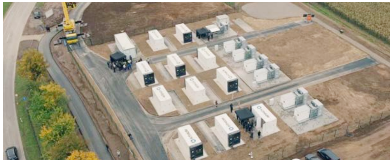
Building Europe's First Large-scale Grid-forming Energy Storage Project
