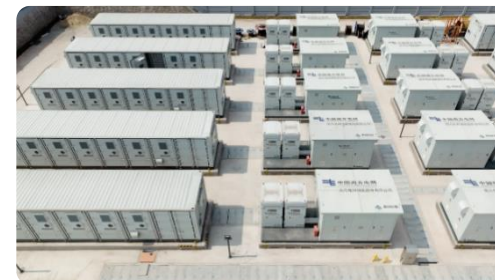
Guangdong, China 70MW / 140MWh
