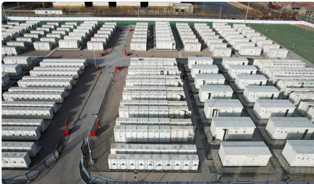
Ningxia, China 200MW / 400MWh
