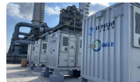
Zhejiang, China 10MW / 20MWh
