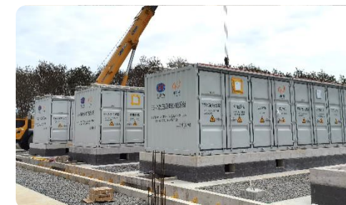
Hainan, China 25MW / 50MWh
