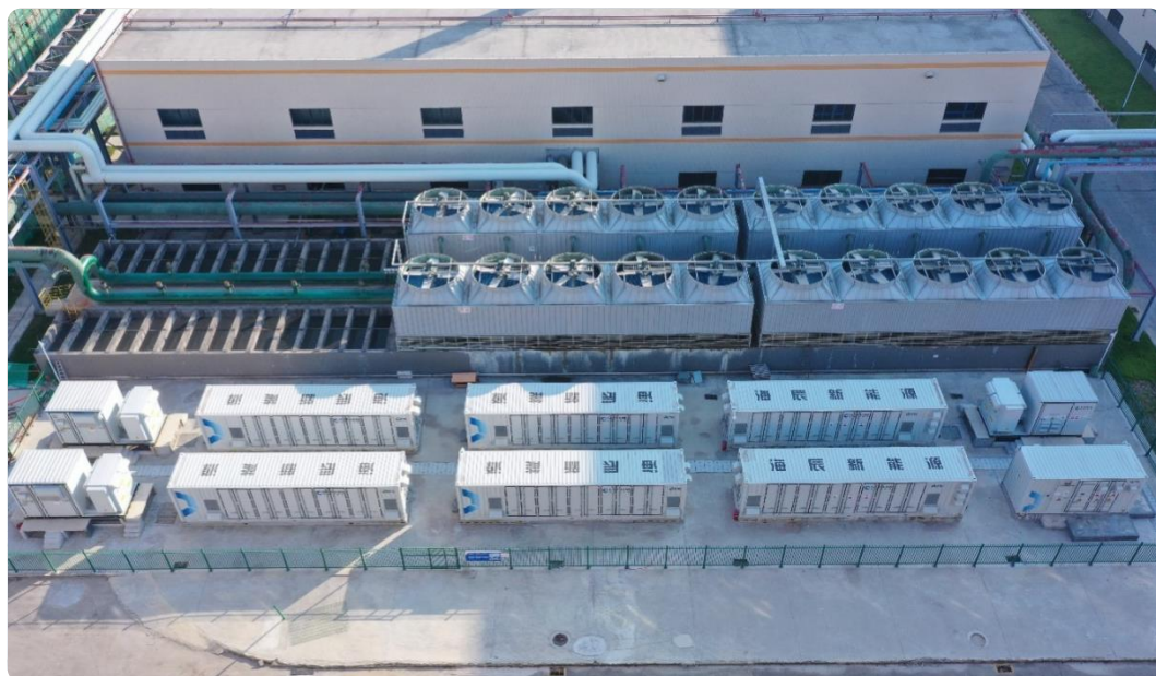
Guangdong, China 7.5MW / 21.5MWh
